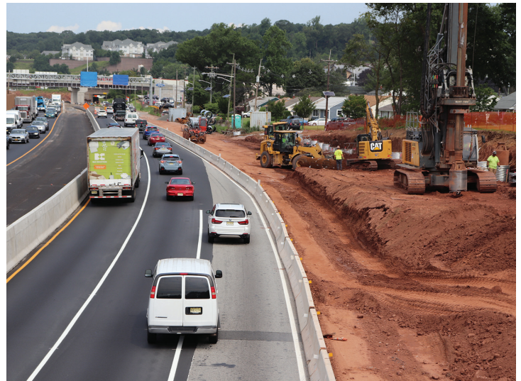
Pictured: Route 3/Route 46 Valley & Notch Road Interchange project site in Clifton, New Jersey.
