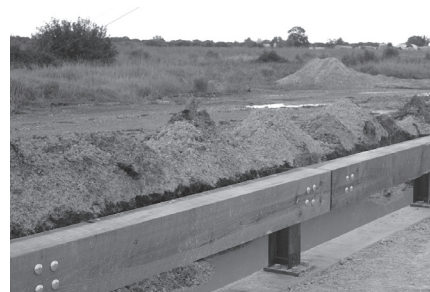
Steel backed timber guide rail provides aesthetic appeal while ensuring safety (Source: Malcom Ray, civil-ws2.wpi.edu/Documents/Roadsafe/Guides ).
