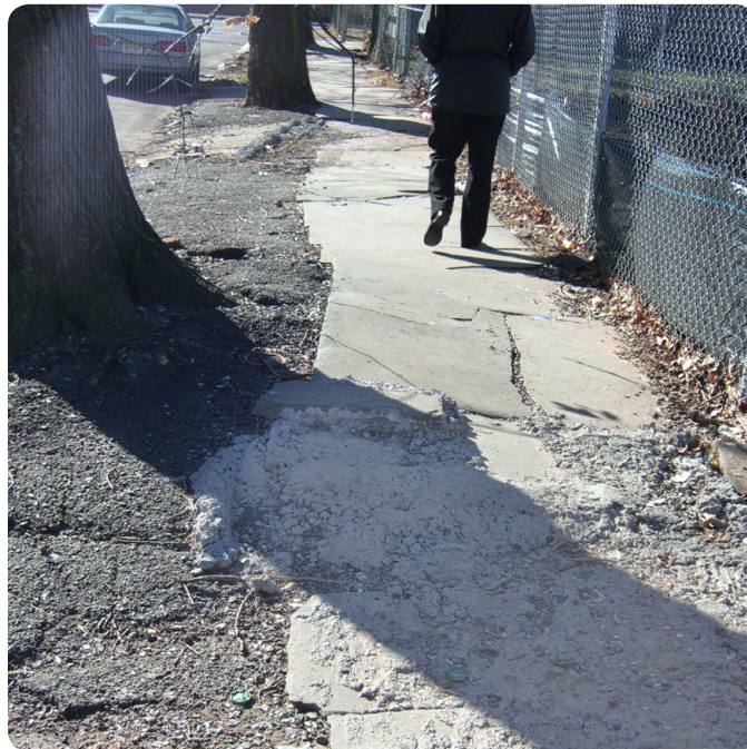
Poor example: This poorly maintained sidewalk is a hazardous impediment for pedestrians and is likely impassable for a wheelchair. It sends the message that this space is not cared for. Image: The RBA Group
