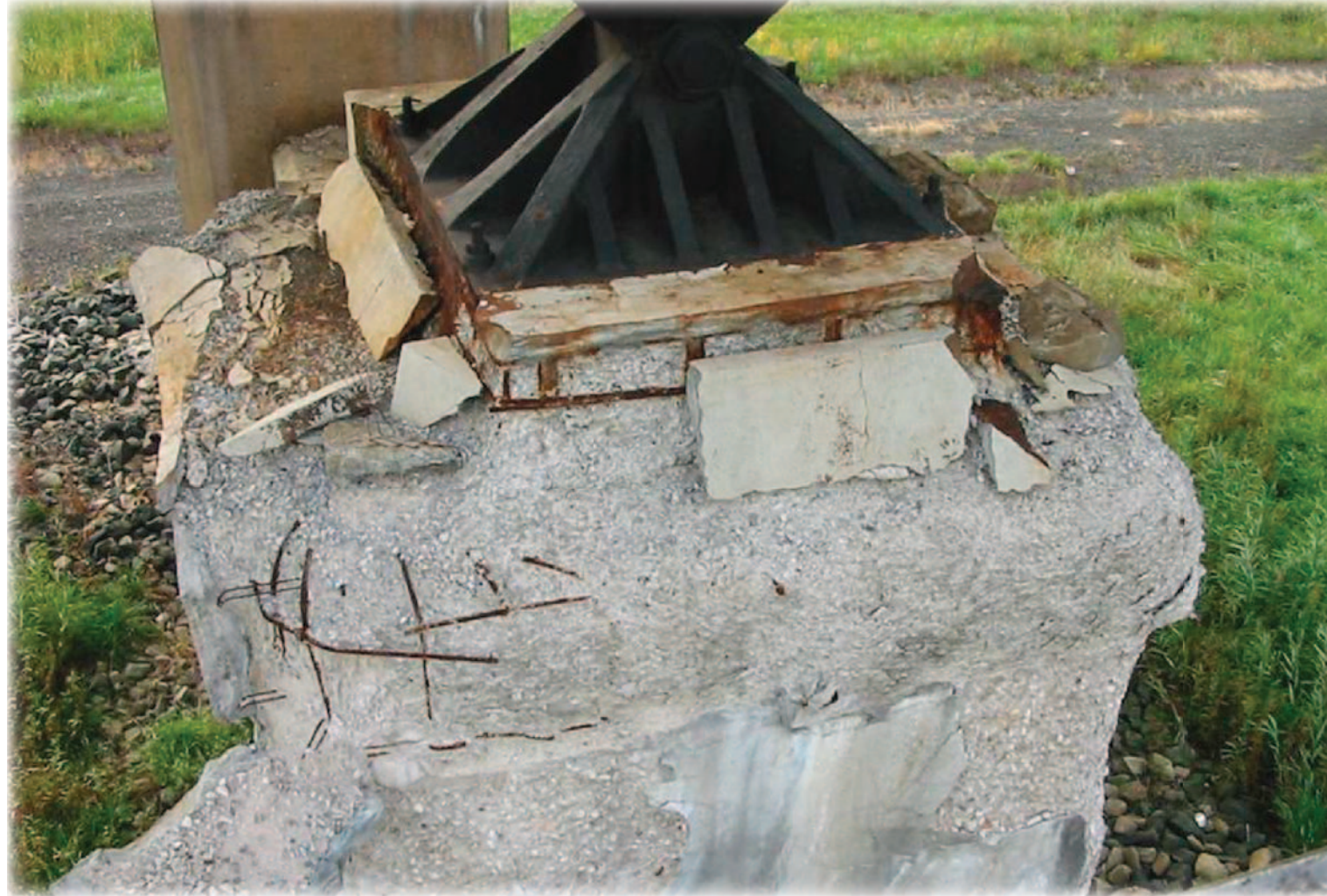
Deterioration on top of concrete column
