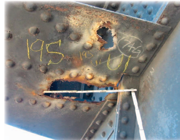
Deterioration of structural steel
