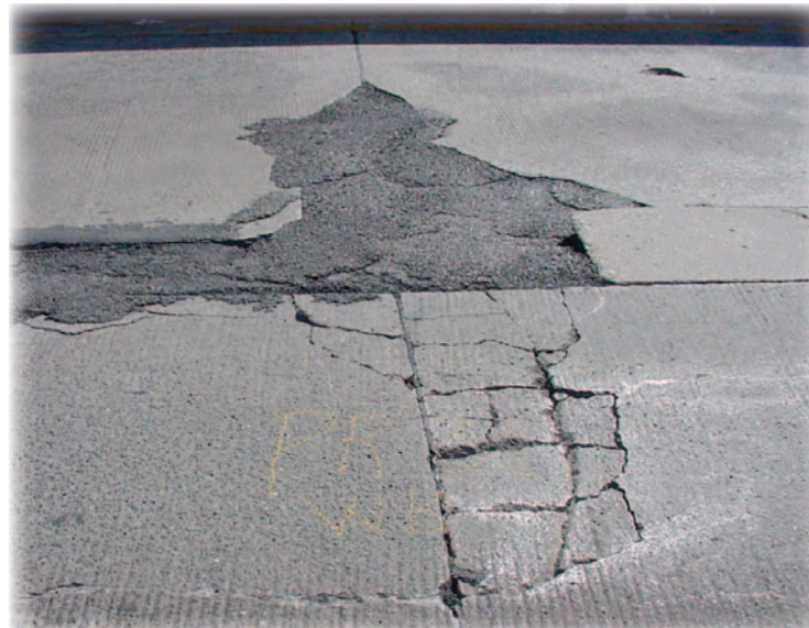
Roadway deck cracking and deterioration
