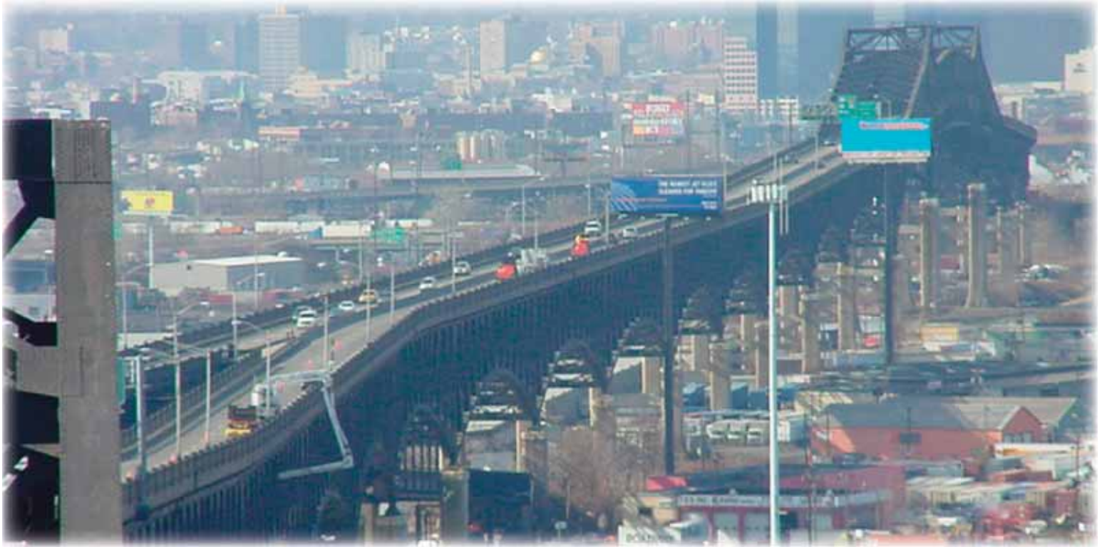
The Skyway rises high above the Meadowlands, reaching a height of over 135 feet. It is included in the National Register of Historic Places because of its age and unique design features.
