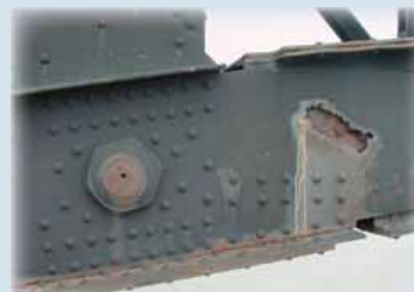
Steel corrosion to be addressed in future repair project.
