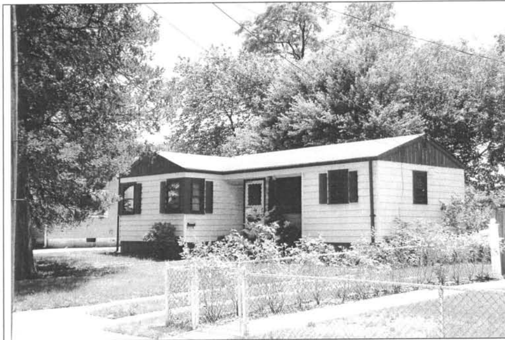
Photograph 2: 307 Grant Avenue. Note the modern replacement windows and vinyl siding. View looking west (May 2004).
