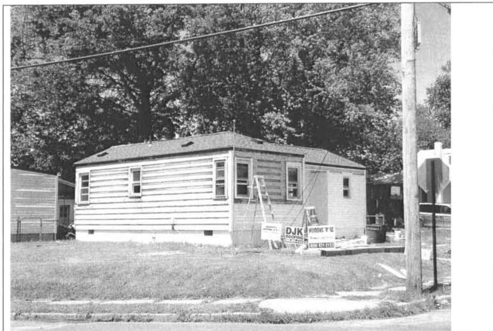
Photograph 3: Northwest corner of Winthrop and Grant avenues. Note the original clapboard siding. Replacement windows, doors, and siding are currently being applied. View looking northwest (May 2004).
