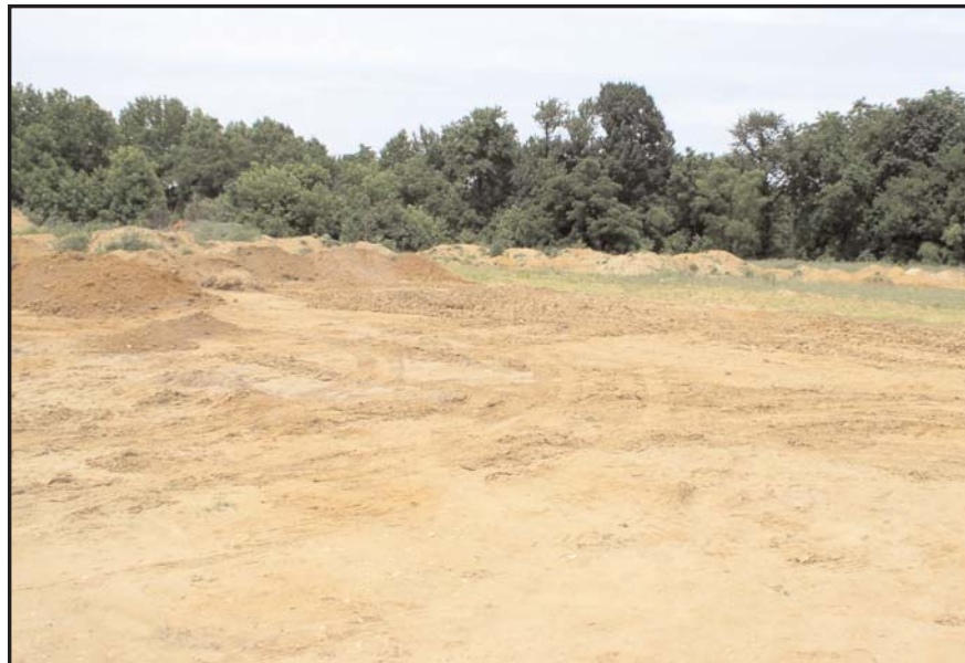
Plate 2: Stockpiled soil in the center of Area I. View looking northwest (June 2004).
