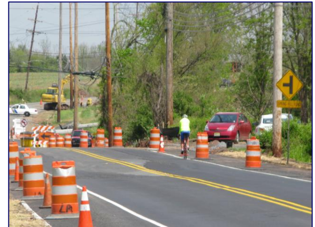
This rural arterial highway under construction in Somerset County incorporates Complete Streets elements and sustainable stormwater management.
