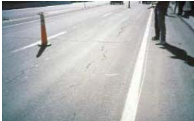
Low Severity Wheelpath
