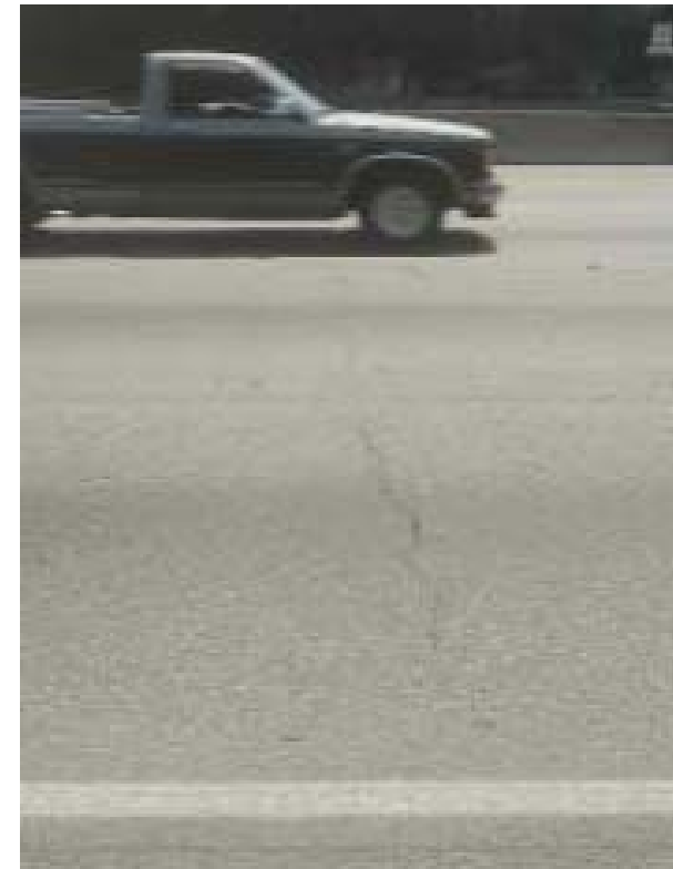
Low to Mod. Transverse Cracking
