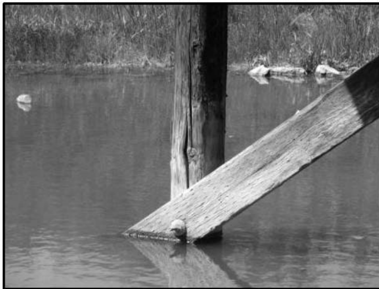
Figure B4.4 – 7 inch deep check in right exterior pile of Bent 2
