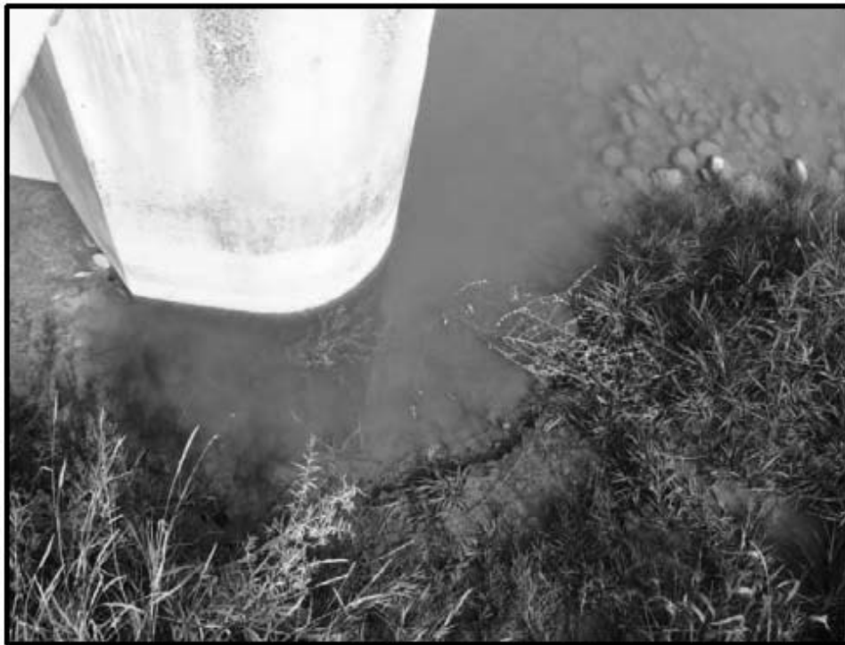
Figure B-6.7: Scour hole at the upstream end of the Pier Wall
