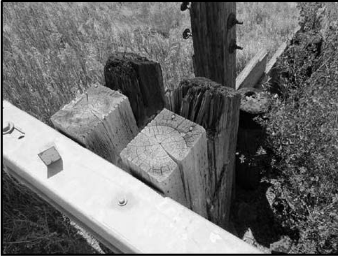
Figure B4.5: Decay in timber rail posts
