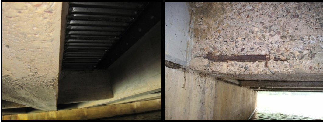
Figure B1.5—Typical Concrete Encasement Condition (Left), Localized Spalling of Concrete Encasement (Right)
