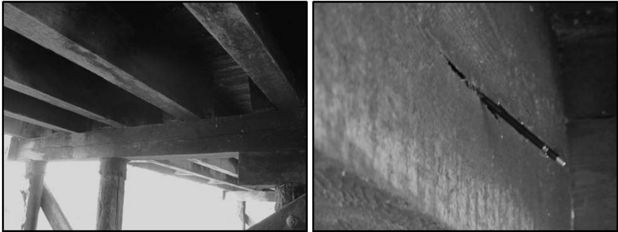
Figure B4.3 – 1 inch deep check in bent cap at Bent 2
