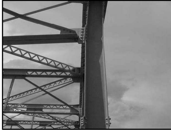
Figure B6.3: Sway bracing impact damage in Span 1
