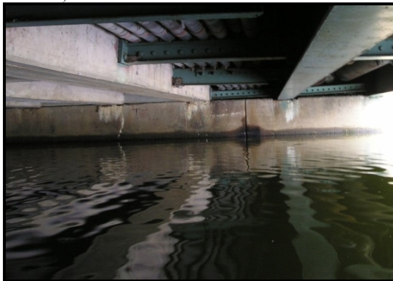
Figure B1.6—Typical Efflorescence Staining
