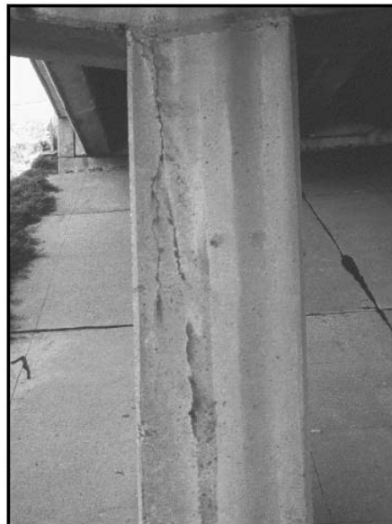
Figure B5.7: 3/16 in. width vertical crack in left column of Pier 4
