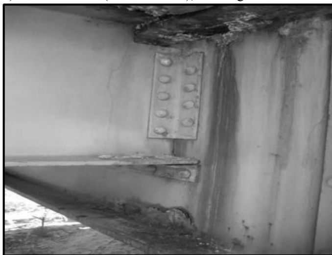
Figure B6.5: Corrosion at floor beam ends
