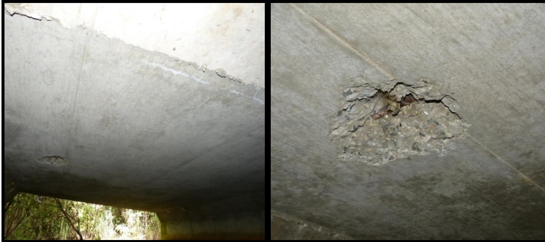
Figure B3.2—Spalls with exposed Rebar at Roof Slab.
