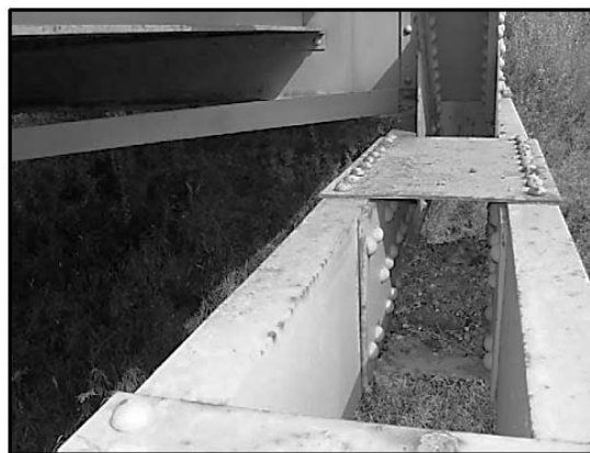
Figure B6.4: Freckle rust, typical, both trusses, both spans
