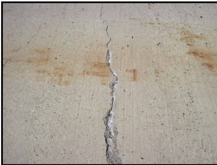
Figure B1.2 –Wide Transverse Crack on Approach Slab
