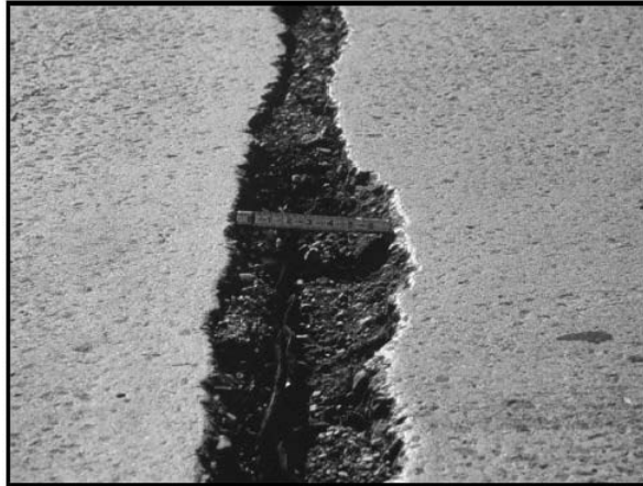
Figure B5.4: Deep spalls in the deck adjacent to the joint seal at Pier 3
