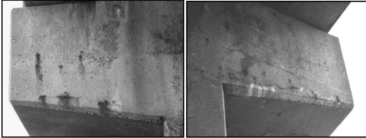
Figure B5.6: 0.04 in. width cracks with rust staining in the cantilevers of the Pier 3 cap
