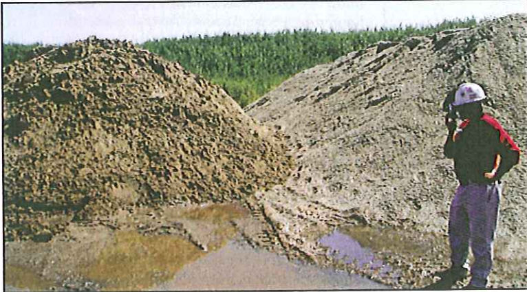
Captain Jeff Bacon of the Corps of Engineers, Philadelphia District photographs piles of sand, left, and crushed recycled glass called cullet that will be combined to create fill material for road construction. Photo by Stanley White, OCC.
