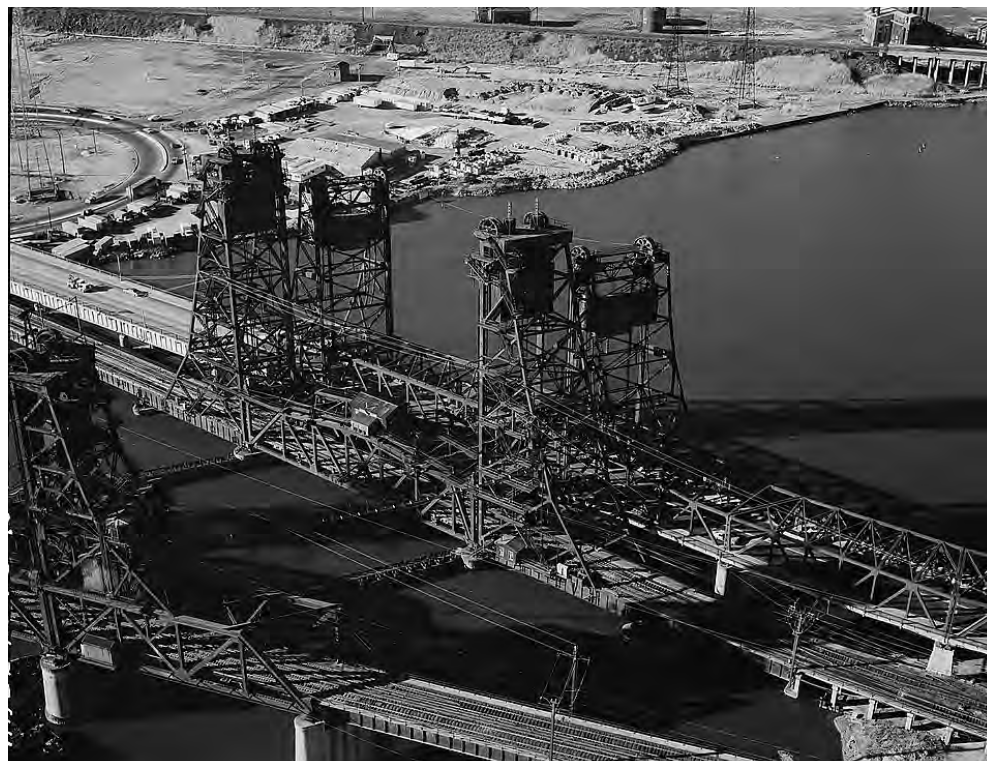
Top: The Pennsylvania Railroad's passenger bridge in 1948. The Port Authority of New York & New Jersey began running PATH trains over the bridge in 1962 (Boucher, HAER-PATH Transit System Bridge).
