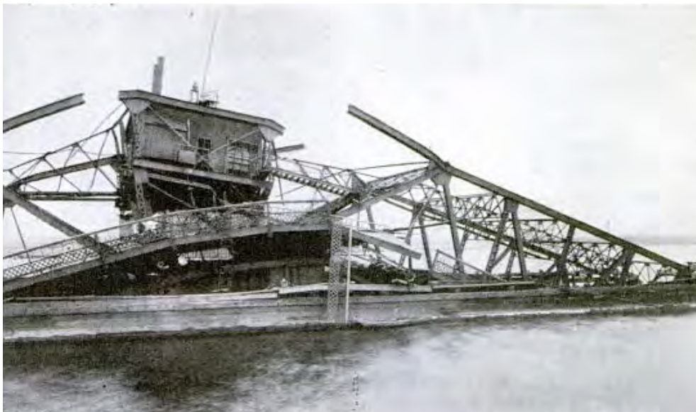
In 1922, the Glendaruel , a steamer loaded with coal making a delivery to the Seaboard By-Product Coke Company crashed into the Lincoln Highway bridge. A temporary bridge was erected within a few months ("Steamer Runs into Open Drawbridge and Wrecks it").
