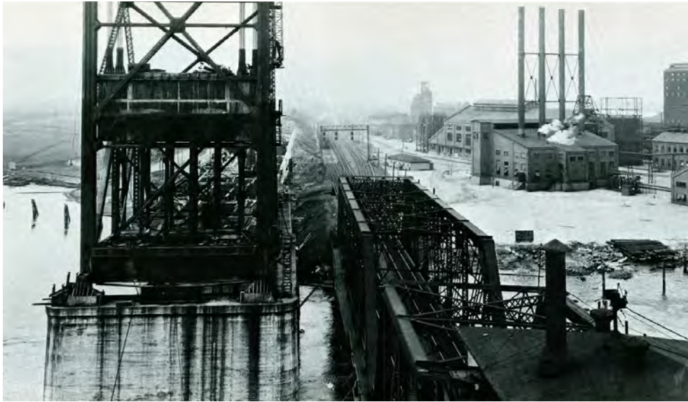
Construction of the new DL&W vertical lift bridge is underway in this circa 1927 photograph. At right are the DL&W's swing span bridge and the Seaboard By-Product Coke Company (Taber).
