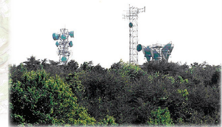
Cell phone towers have become a common feature in the built environment.
